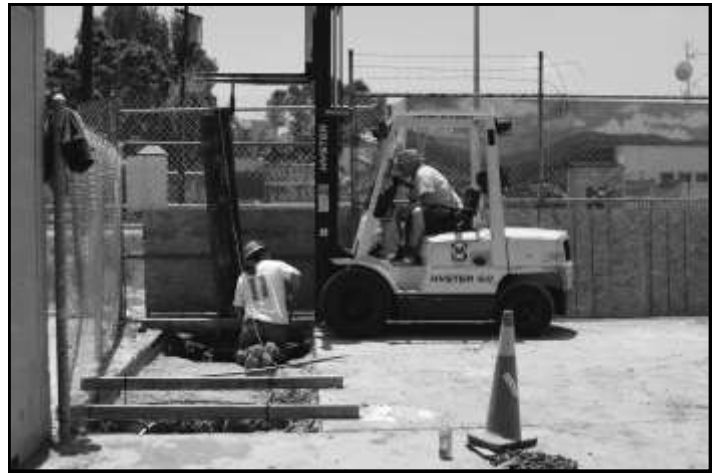
WCHA is lucky to have a Teamster onboard! Jim Danno maneuvers one of the 1' x 14' steel support pipes into place.
